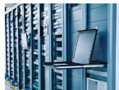
Control Room/ Data Center
