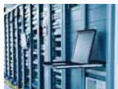
Control Room/ Data Center
