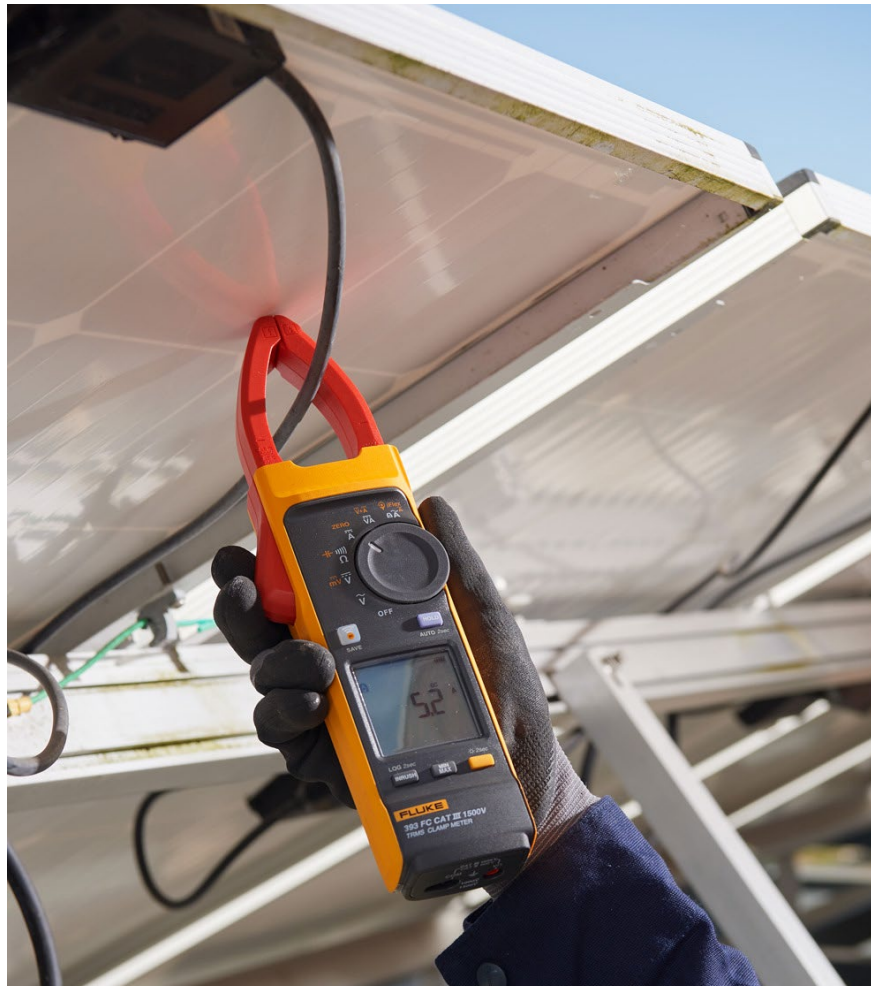
Measuring current on a PV panel with a Fluke 393 FC clamp meter.
