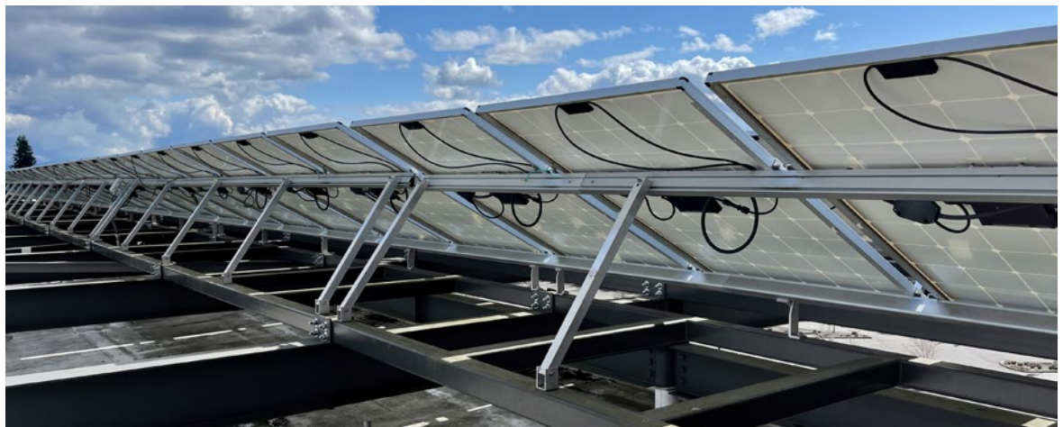
If you work on PV panels, you should know how to work with a non-load break rated disconnect.
