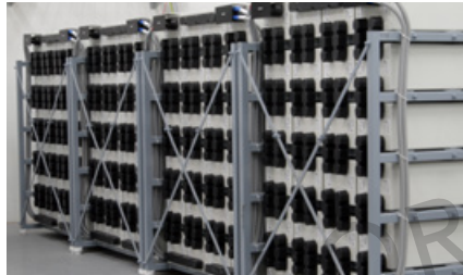
Energy Storage System
