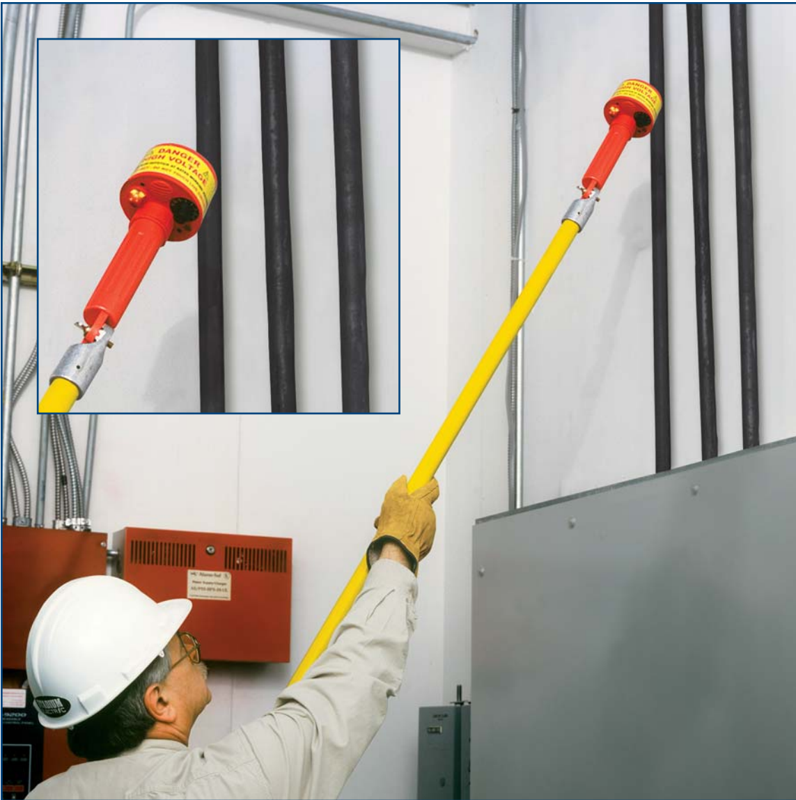
Model 275HVD checking for live voltage on main feeder
